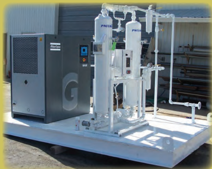
ATLAS COPCO AIR COMPRESSORS
